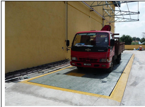
Pit Weigh Bridge
